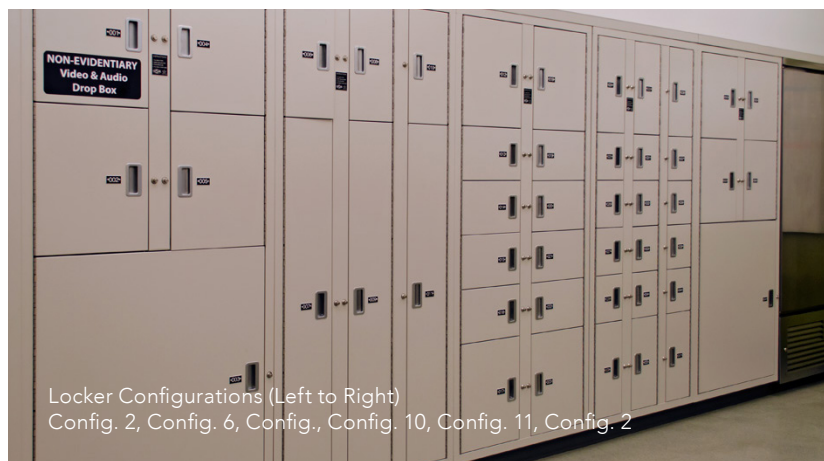
Multiple rows of Locker configuration 15 with full size refrigerators along the back wall at Wake County Detention Center
